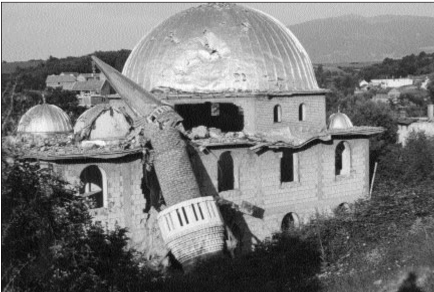
A damaged mosque on the road between Djakovica and Prizren, July 1999.
